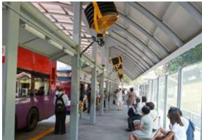
Figure 9: Electric fans installed at the bus stop in Singapore
