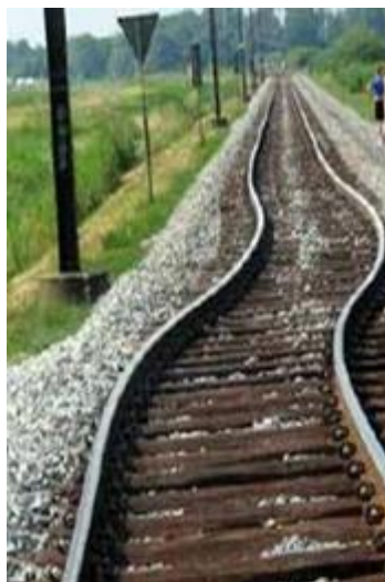
Figure 6: Sun kinks occur with wooden ties
