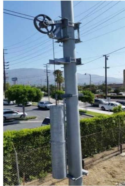
Figure 15: Existing weight stack tensioning system
